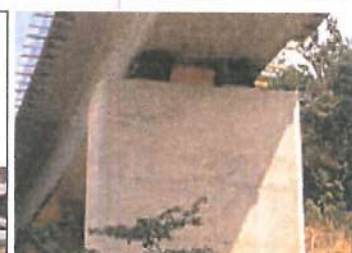
Structural Base Isolator, Hyogo, Japan
